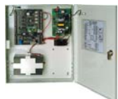
ELEVATOR384 (ELEVATOR CONTROLLER)
